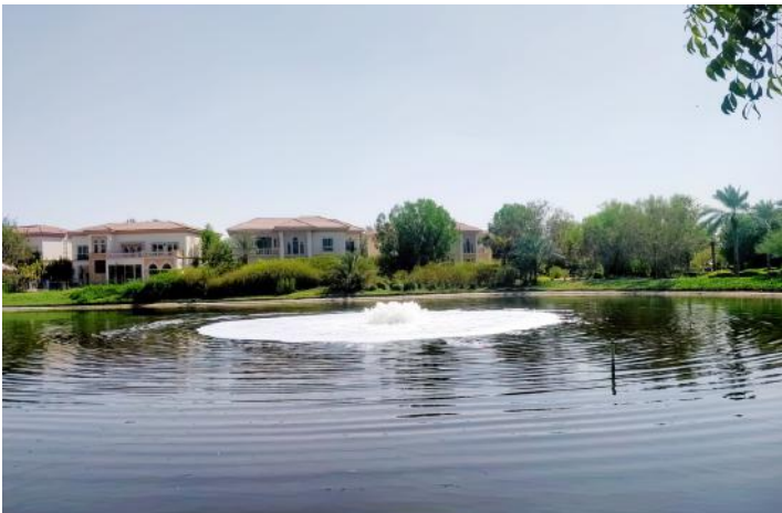
Continued installation of high volume, sunburst and subsurface aeration systems across the 19 lakes. Completion of aerators installation expected by end of October.
